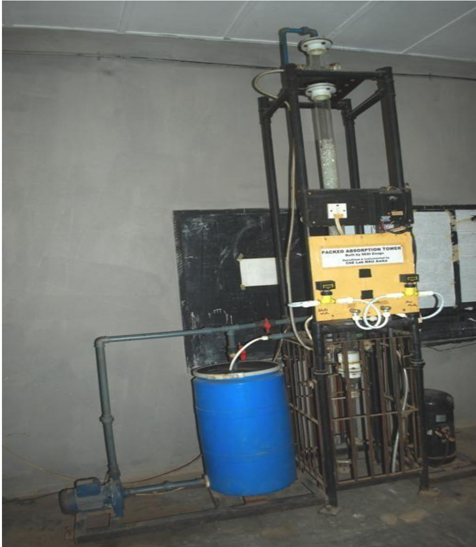
FigureH-1: The photograph of the prototype pilot plant packed absorption tower after retooling with electronic rotameters and manometer.
